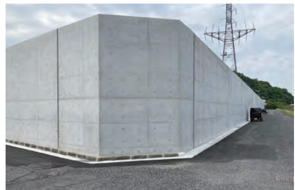
高陽取水場の防水壁 Flood barriers at Koyo Intake Station
